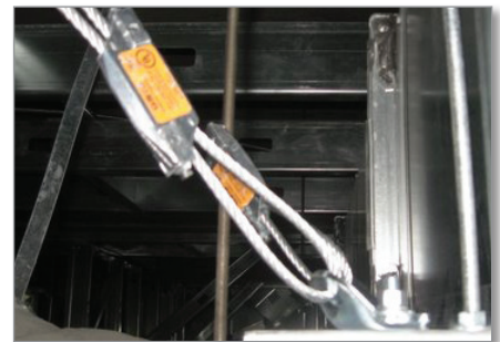
Bracing of rectangular ductwork
