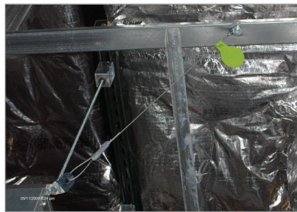
Bracing of busduct
