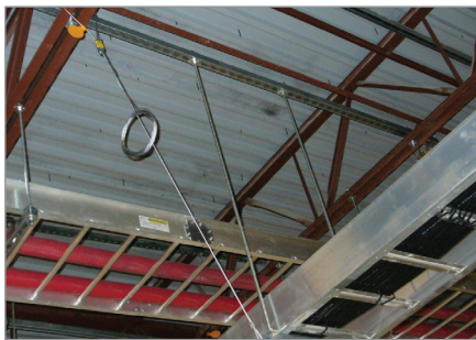
Bracing of electrical services
